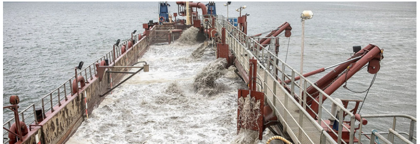
Ships dredging sand from the seabed at Port Esbjerg to deepen the fairway.
